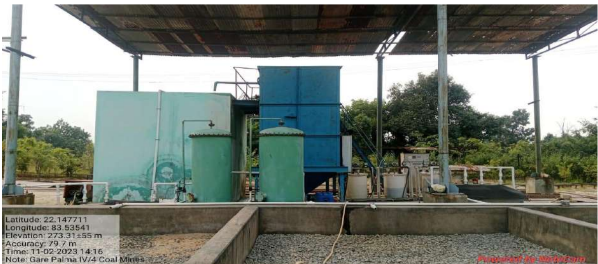
Effluent Treatment Plant – 50 KLD - Bankheta
